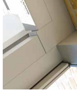
Waterafvoer via goot direct in steunpaal
