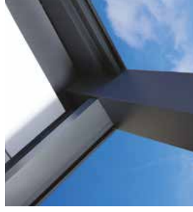
Waterafvoer via goot direct in steunpaal
